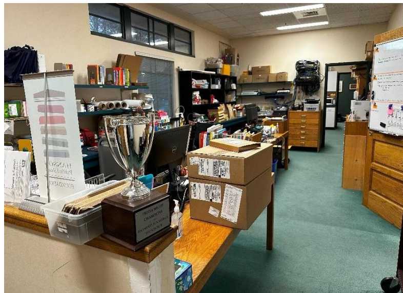
Staff Workroom with network equipment mounted in the open on the far wall
