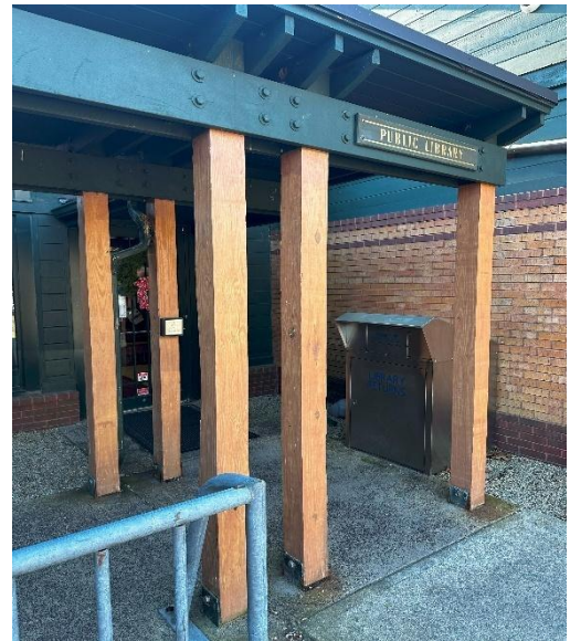
Entryway to shared lobby, Library entrance, community meeting room, and external book return
