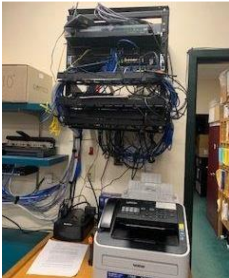
Network equipment on open shelving in Staff Workroom
